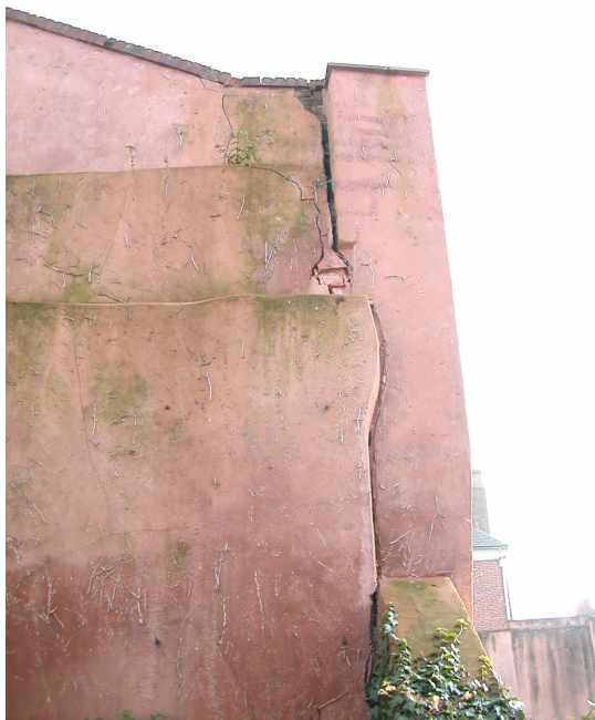
Crack in wall to rear of 144 Fore Street, overlooking car park of Homecourt House
